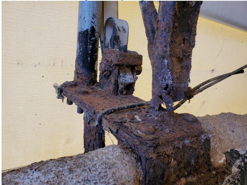
Figure 2: Damage to structural elements due to salt buildup on top of low interior walls
