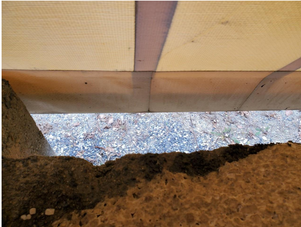
Figure 3: Gap between wall and cover. The current wall is too low, allowing salt to spill over the top and escape the structure through the gap between the cover and wall. From there, stormwater carries the salt to the Black River.
