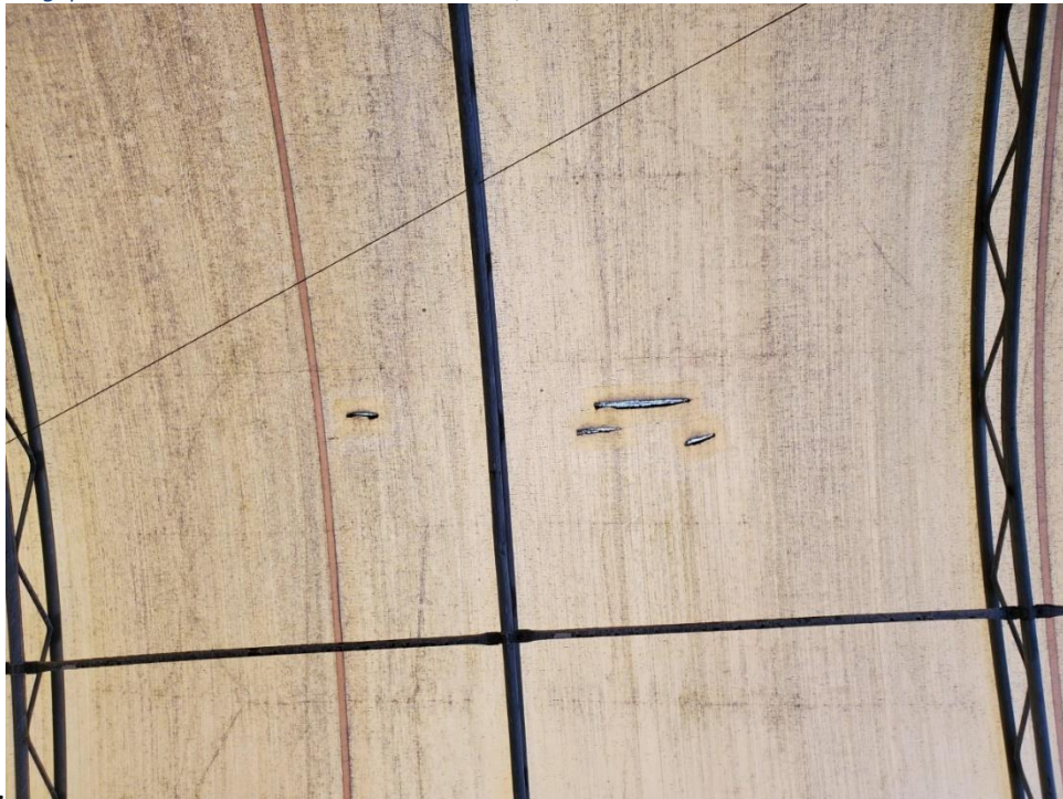
Figure 4: Damage to existing cover allowing stormwater to infiltrate the structure and carry away road salt.
